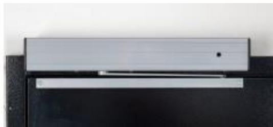
Automatic Door Opening
